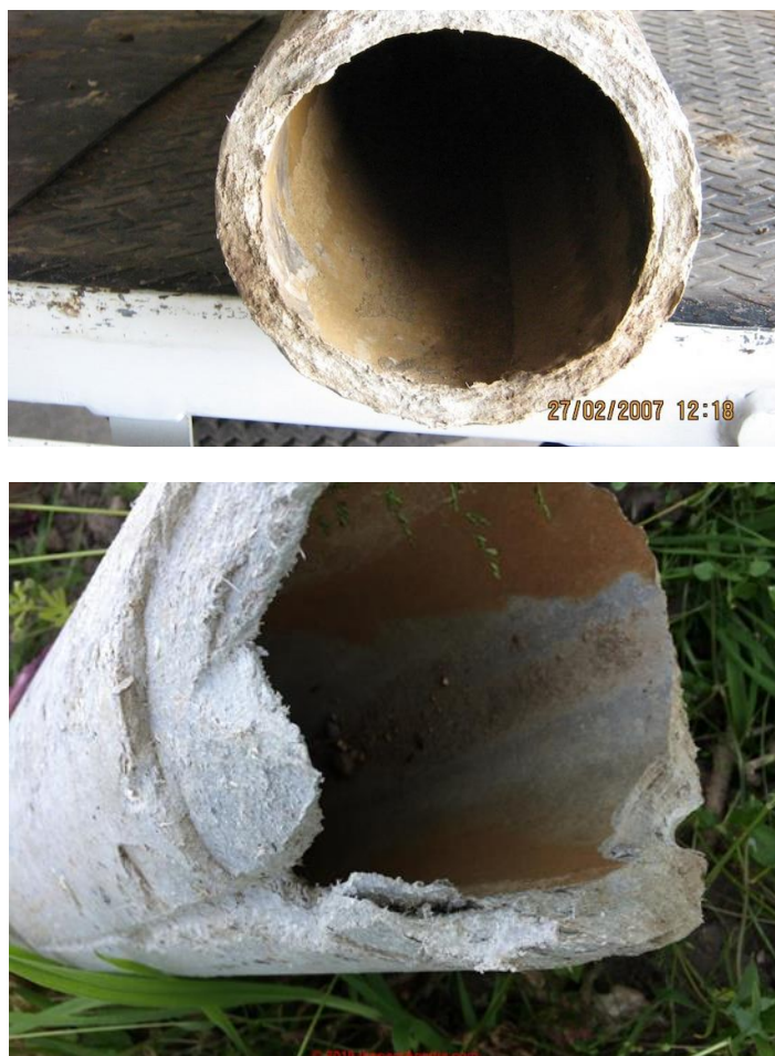
Figure 6:Old Water Pipes
